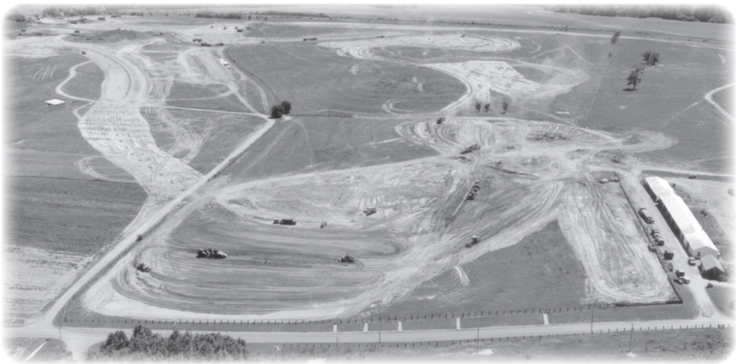
In September 1988, the Missouri National Guard completed work to bring the land up to grade for the Patrol's Defensive Driving Track.
