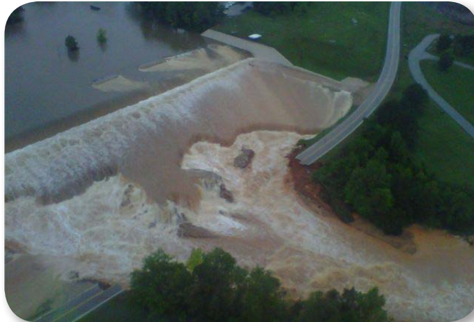
Flood waters breached the emergency spillway of Wappapello Dam and washed out approximately 400 feet of Missouri Route T. Locals now refer to this area as the Little Grand Canyon.
