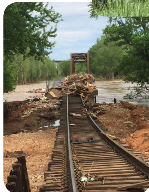
The railroad bridge at Jerome, MO, sustained extensive damage from the spring flood waters.
